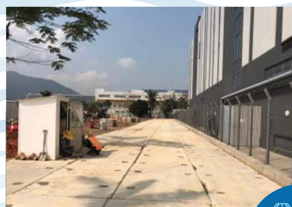
以可重用的混凝土、含瀝青的硬填料或金屬板覆蓋臨時通道，避免塵土飛揚 Temporary access are paved with reusable concrete, bituminous hardcore materials or metal plates to minimise dust generation
