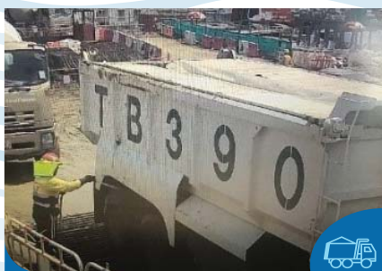
運送易生塵埃物料的車輛在離開工地前必須蓋上機械蓋掩或防水布 Vehicles transporting dusty materials must be covered by mechanical cover or tarpaulin sheets before leaving the site
