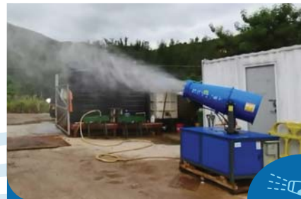
使用自動噴霧器保持建築物表面及工地濕潤 Using automatic mist sprayer to dampen the surface of construction materials and the site
