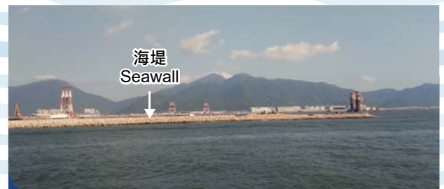
進行海上填料工程前先建造至少200米長的前緣海堤 An advance seawall of at least 200m was constructed prior to the commencement of marine filling activities
