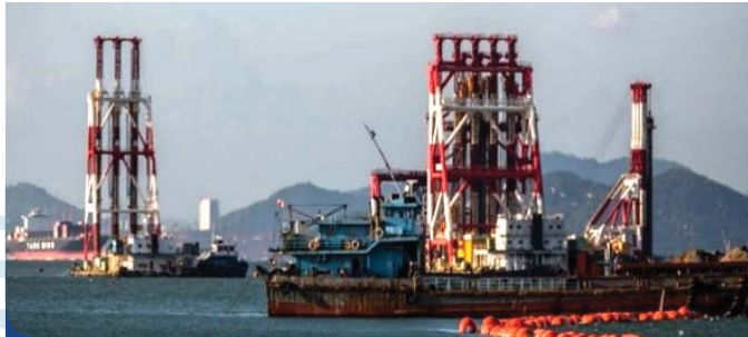
使用免挖式的深層水泥拌合法在污染泥料卸置坑範圍進行地質改善工程 Use of non-dredge Deep Cement Mixing (DCM) as the ground improvement method at the contaminated mud pit areas
