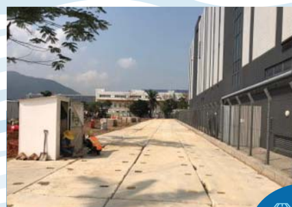
以可重用的混凝土、含沥青的硬填料或金属板覆盖临时通道，避免尘土飞扬 Temporary access are paved with reusable concrete, bituminous hardcore materials or metal plates to minimise dust generation
