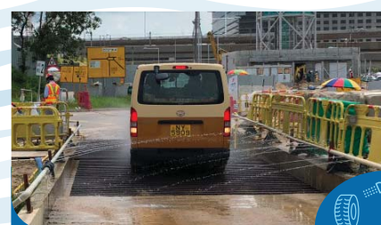
在工地出口安装车轮清洗设施为车辆的轮胎除去尘埃 Install wheel washing facilities at construction site exit to wash off dust from wheels of vehicles
