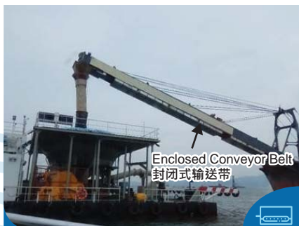
使用封闭式输送带运送填料 Using enclosed conveyor belt to transport fill materials
