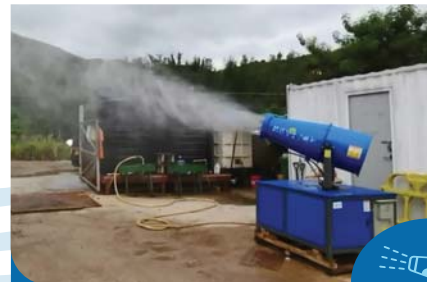
使用自动喷雾器保持建筑物表面及工地湿润 Using automatic mist sprayer to dampen the surface of construction materials and the site
