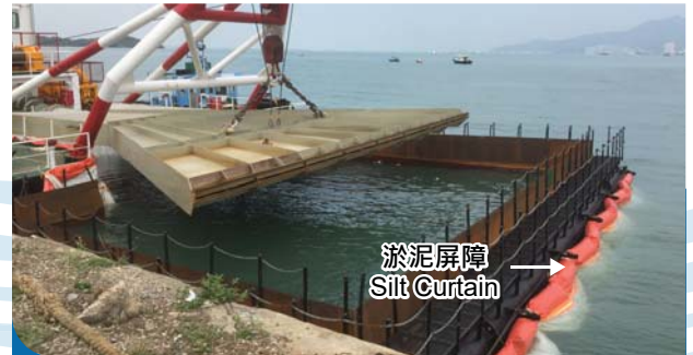
铺设砂垫层时设置笼式淤泥屏障 Deployment of localised cage-type silt curtains for sand blanket laying activities
