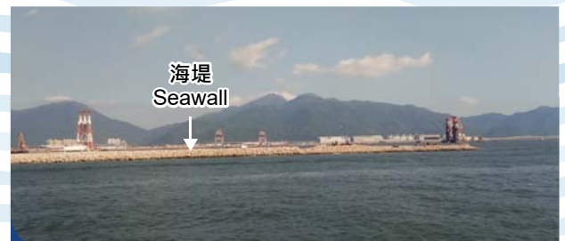
进行海上填料工程前先建造至少200米长的前缘海堤 An advance seawall of at least 200m was constructed prior to the commencement of marine filling activities
