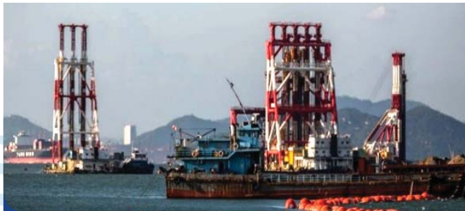
使用免挖式的深层水泥拌合法在污染泥料卸置坑范围进行地质改善工程 Use of non-dredge Deep Cement Mixing (DCM) as the ground improvement method at the contaminated mud pit areas
