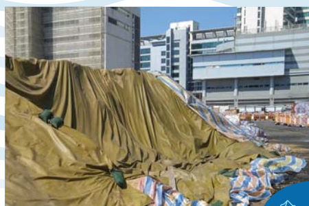
以不滲透的隔塵布覆蓋儲料區 Covering stockpiling areas with impervious sheets
