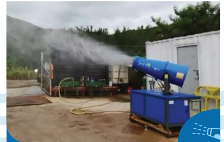
使用自動噴霧器保持建築物表面及工地濕潤 Using automatic mist sprayer to dampen the surface of construction materials and the site
