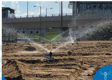
以360度自動花灑定期向填料灑水 Regularly using 360 degree automatic sprinkler to dampen fill materials
