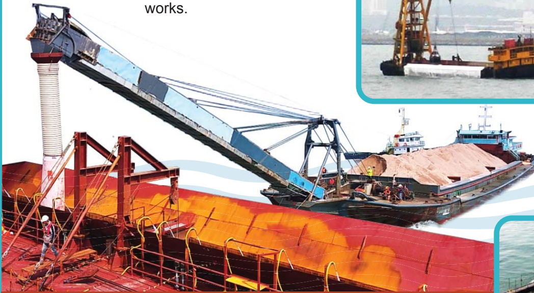
在土工織物防護膜上鋪設砂墊層 Laying of sand blanket on top of geotextile
