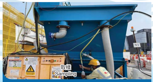
工地的污水在排放前須經污水處理設施處理，並定期由承建商取樣監測，以確保符合《水污染管制條例》的要求 Wastewater discharged from construction site is processed at wastewater treatment facilities and monitored regularly by contractors to ensure compliance with the requirements of the Water Pollution Control Ordinance
