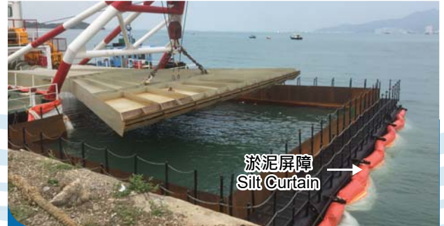
鋪設砂墊層時設置籠式淤泥屏障 Deployment of localised cage-type silt curtains for sand blanket laying activities
