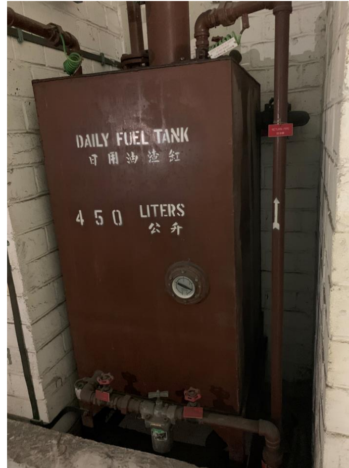
BH7 View 1 - 450 L Above-ground Fuel Tank
