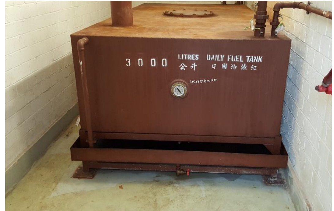
BH9 View 1 - 3000L Above-ground Fuel Tank (BH9)
