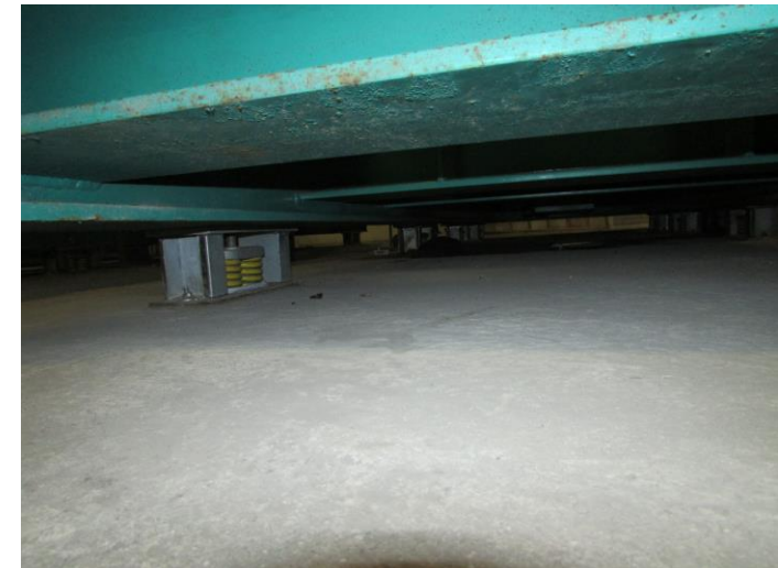
HS1 View 2 - concrete floor condition underneath emergency generators
