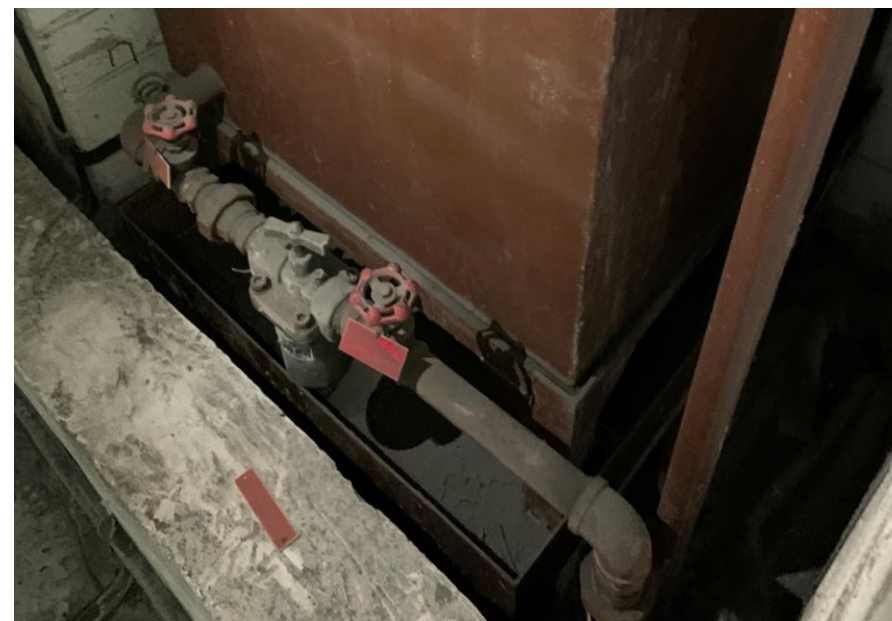
BH7 View 2 – Drip tray condition underneath 450 L Above-ground Fuel Tank
