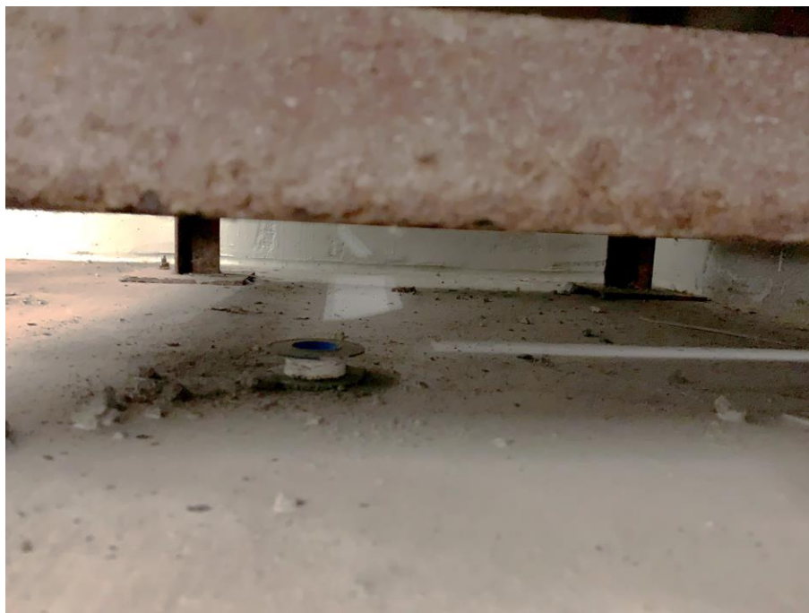
BH3 View 2 – concrete floor condition underneath 450 L fuel tank
