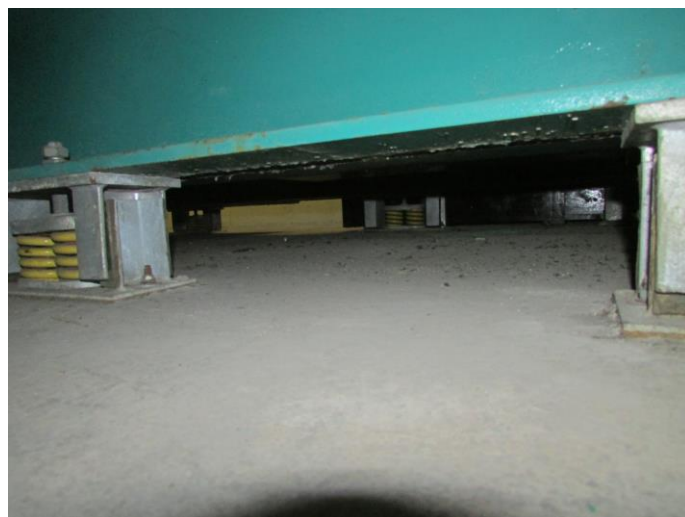
HS1 View 3 - concrete floor condition underneath emergency generators
