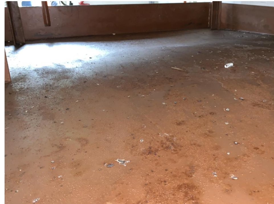
BH10 View 2 - drip tray condition of the 1,500L Above-ground Fuel Tank
