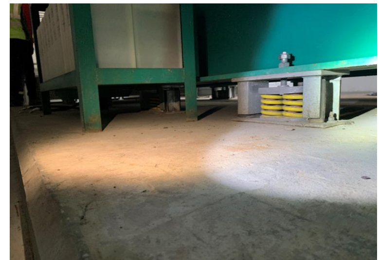
HS2 View 3 - concrete floor condition underneath emergency generator
