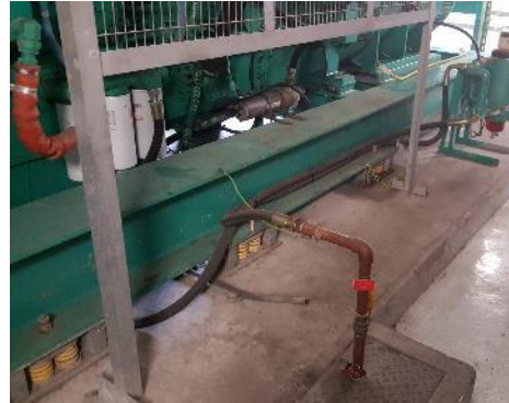
Fuel pipes to/from fuel tank and the generator
