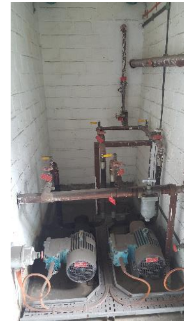
Fuel pump room
