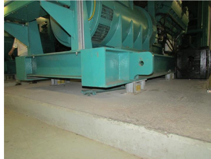
HS1 View 1 - concrete floor condition underneath emergency generators
