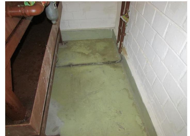
HS4 View 2 - concrete floor condition of fuel tank room with 1,500 L above-ground fuel tank
