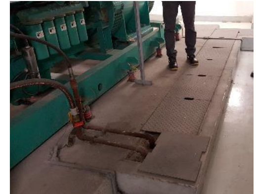
Fuel pipes to/from 450L fuel tank and the generator
