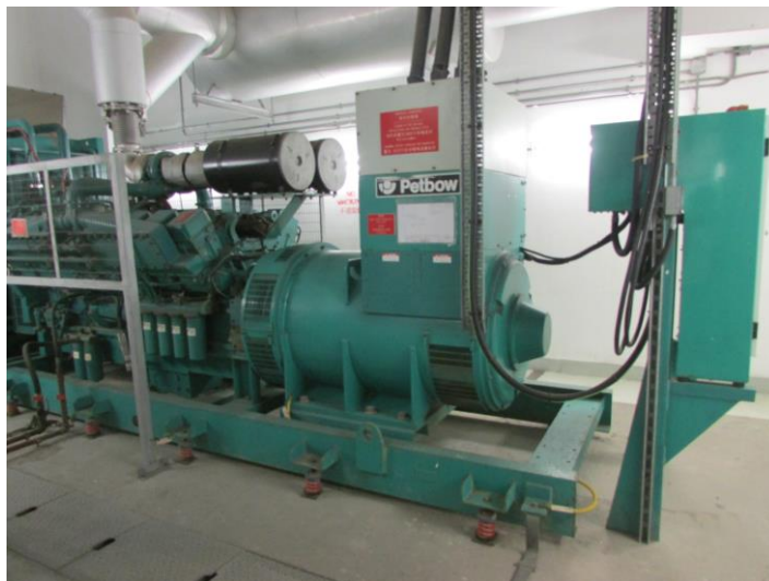
BH4 View 1 - Emergency Generator (BH4) (Mounted on 200mm-thick concrete plinth)
