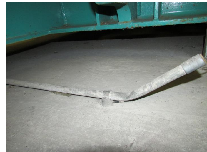
HS1 View 5 - concrete floor condition underneath emergency generators
