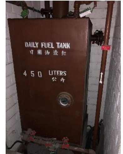
450 L fuel tank (BH7)
