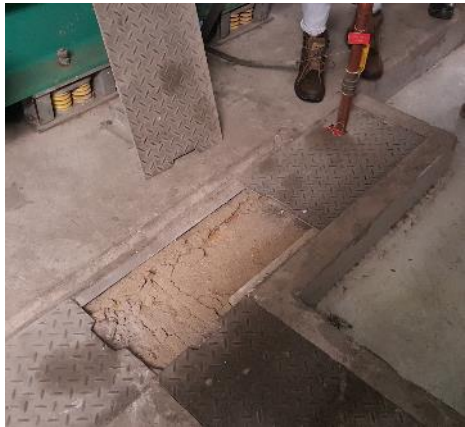
Sand filled trench containing fuel pipes (outside the fuel tank chamber)
