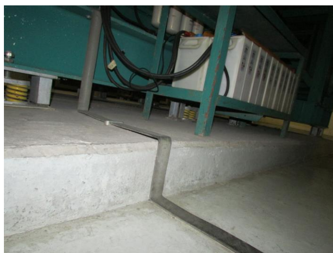
HS1 View 4 - concrete floor condition underneath emergency generators
