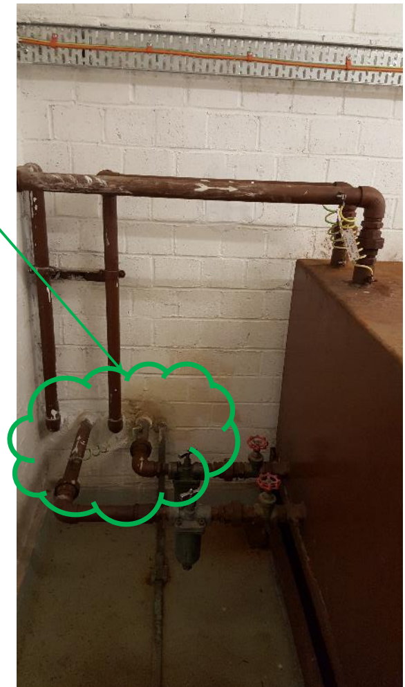
Fuel pipes penetrating the wall and connect to the generators at lower floor
