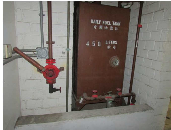
BH7 View 1 - 450 L Above-ground Fuel Tank
