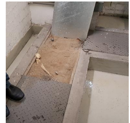
Sand filled trench containing fuel pipes (outside the fuel tank chamber)
