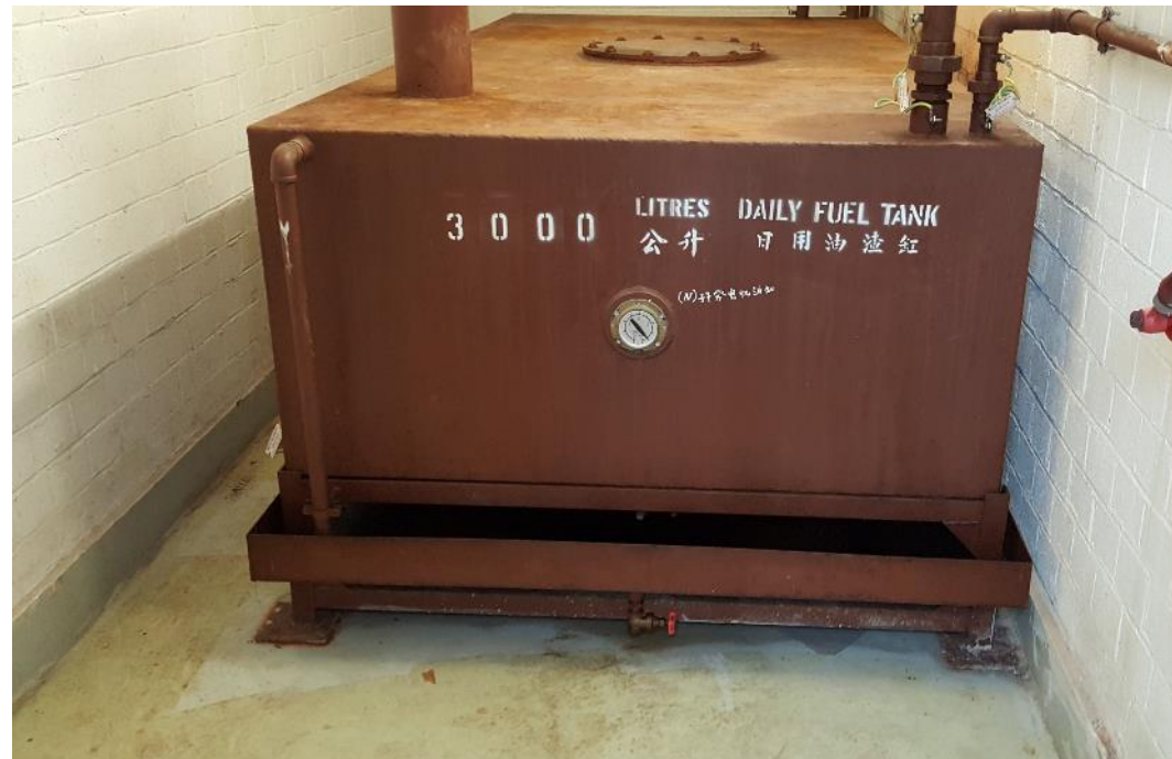
3000 L fuel tank with metal drip tray
