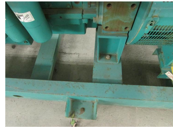
BH4 View 3 - concrete floor condition underneath Emergency Generator
