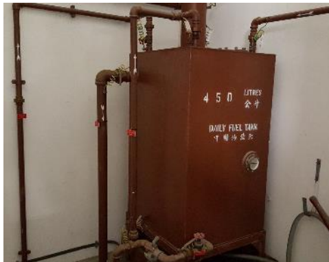
450 L fuel tank (BH3)
