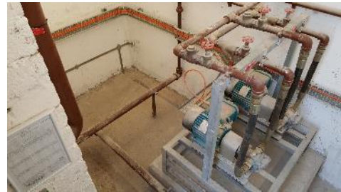
Fuel pump room
