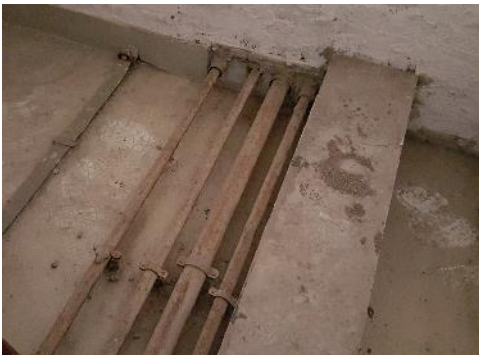
Fuel pipes within the fuel tank chamber (leading to generator BH4)
