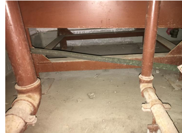
BH3 View 1 – concrete floor condition underneath 450 L fuel tank
