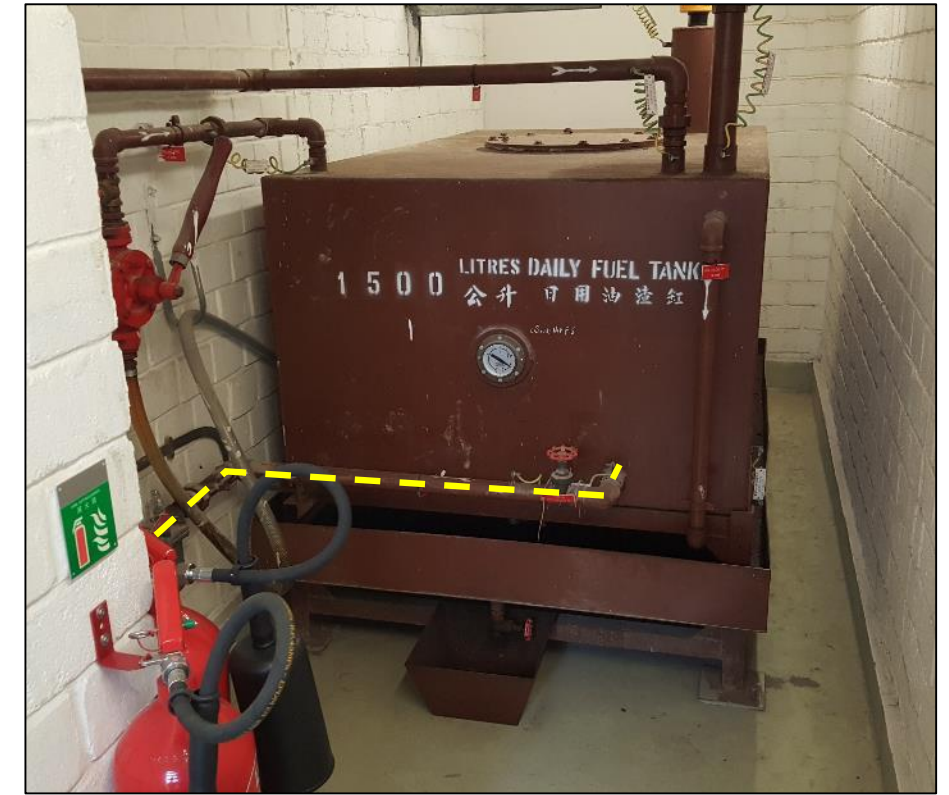
1,500L fuel tank (BH10) with metal drip tray
