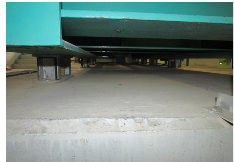
HS2 View 2 - concrete floor condition underneath emergency generator
