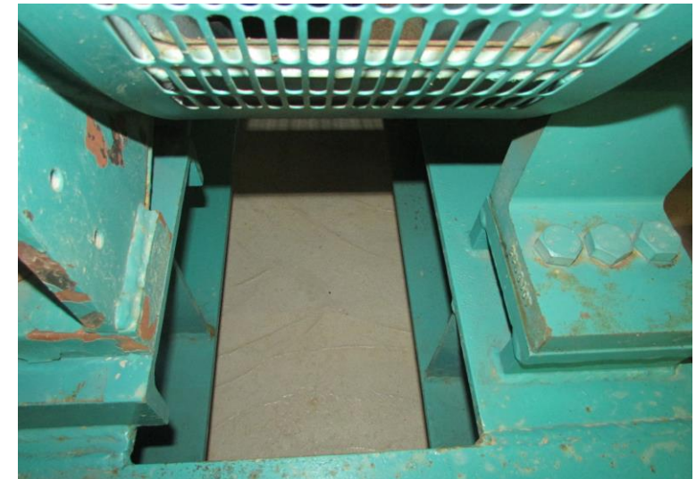
HS2 View 1 - concrete floor condition underneath emergency generator
