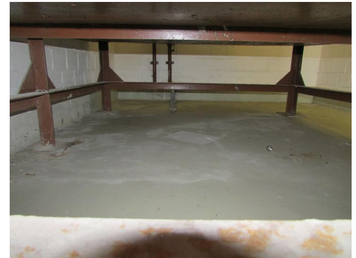
HS4 View 1 - concrete floor condition underneath 1,500L Above-ground Fuel Tank
