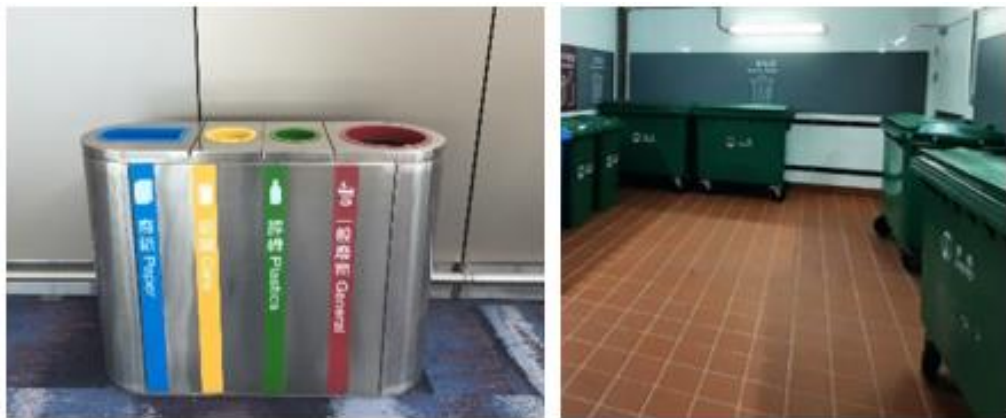
Figure 5.7 Recycling Bin System at HKIA Public Areas (left) and General Refuse Containers with Covers at the Refuse Room of the Passenger Terminal Building (right)
