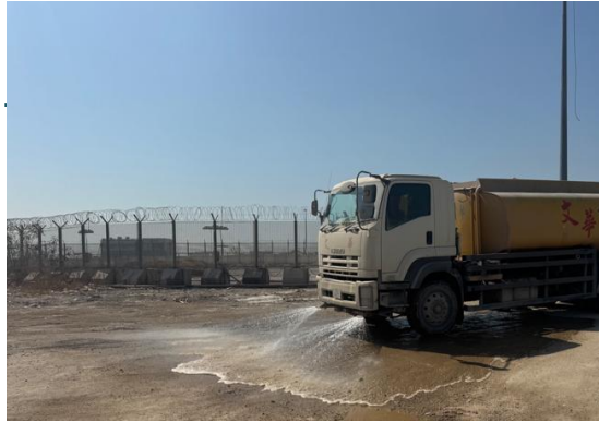
Regular water spraying on main haul roads to minimise fugitive dust emissions
