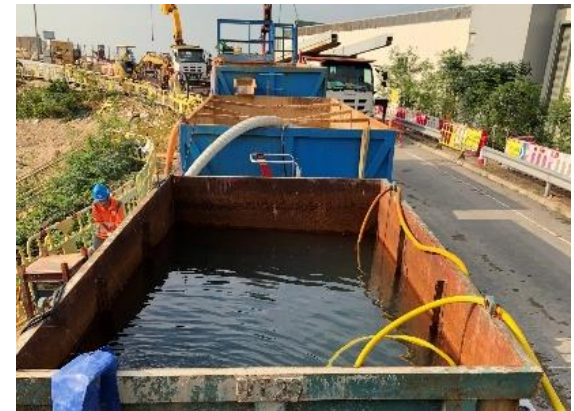
Pre-treatment tanks with coagulant provided to improve silt removal efficiency
