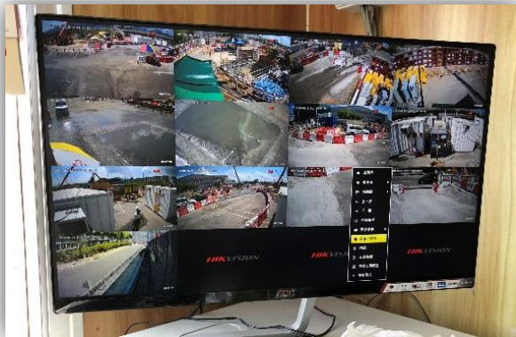
CCTV system as installed at the major vehicular exits of construction site
