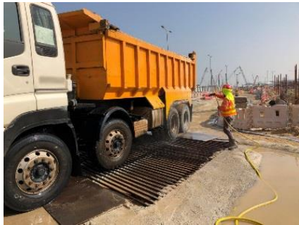
Enhanced wheel washing facility
